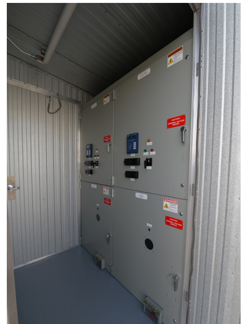
View of Power Control Aisle Interior
