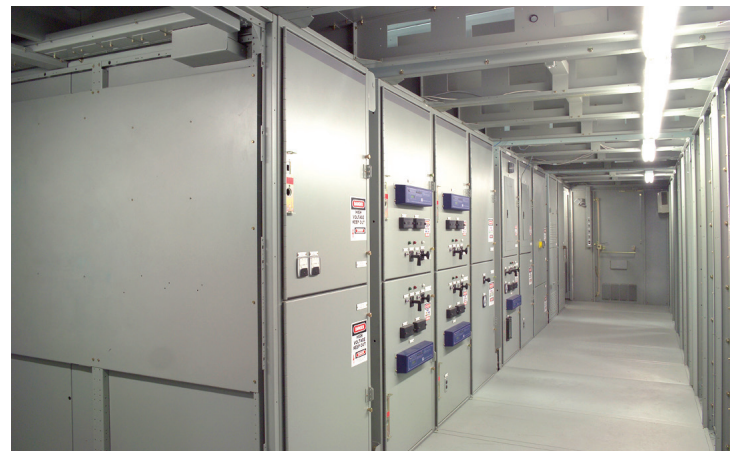
Typical Powell Power Control Aisle™ interior with switchgear installed.
