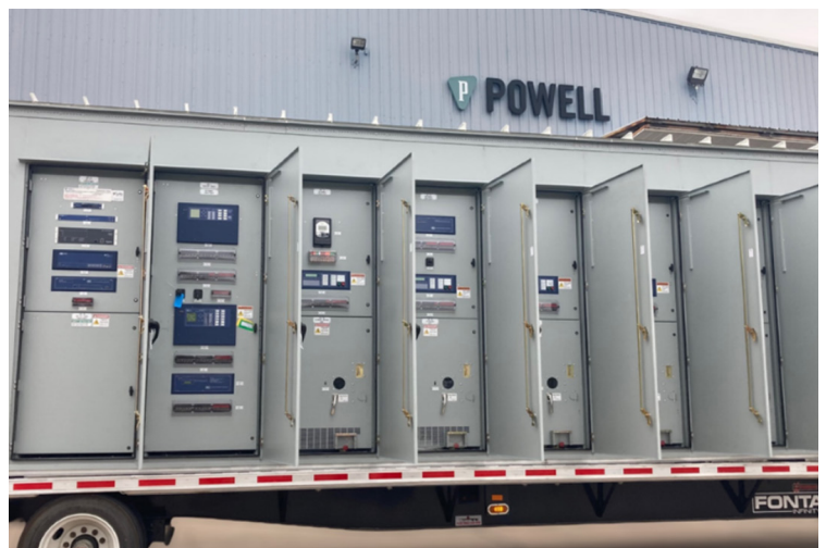
View with exterior weather-proof doors open for breaker/instrument access
